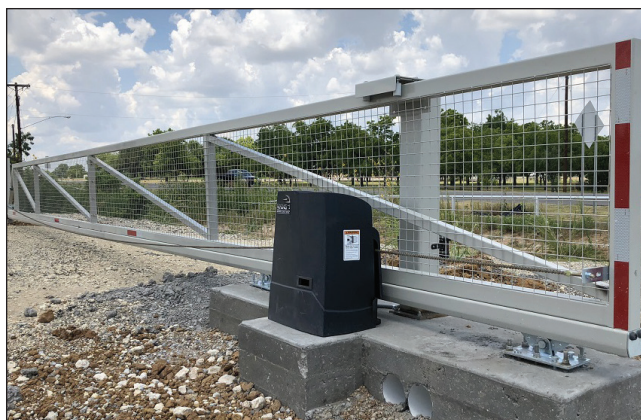
Aberdeen Gates, Weatherford, TX installed a security gate at a local Ford dealer. Model CGS-350.8P was used since the gate opening was large and the gate itself was quite heavy. The gate is fully automated.
